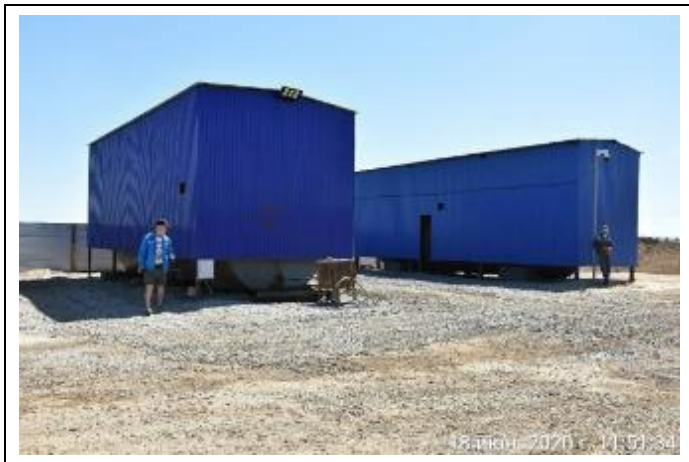
Picture 6. Temporary storage of fuel and lubricant materials within base camp territory, Lot 4. May 2020
