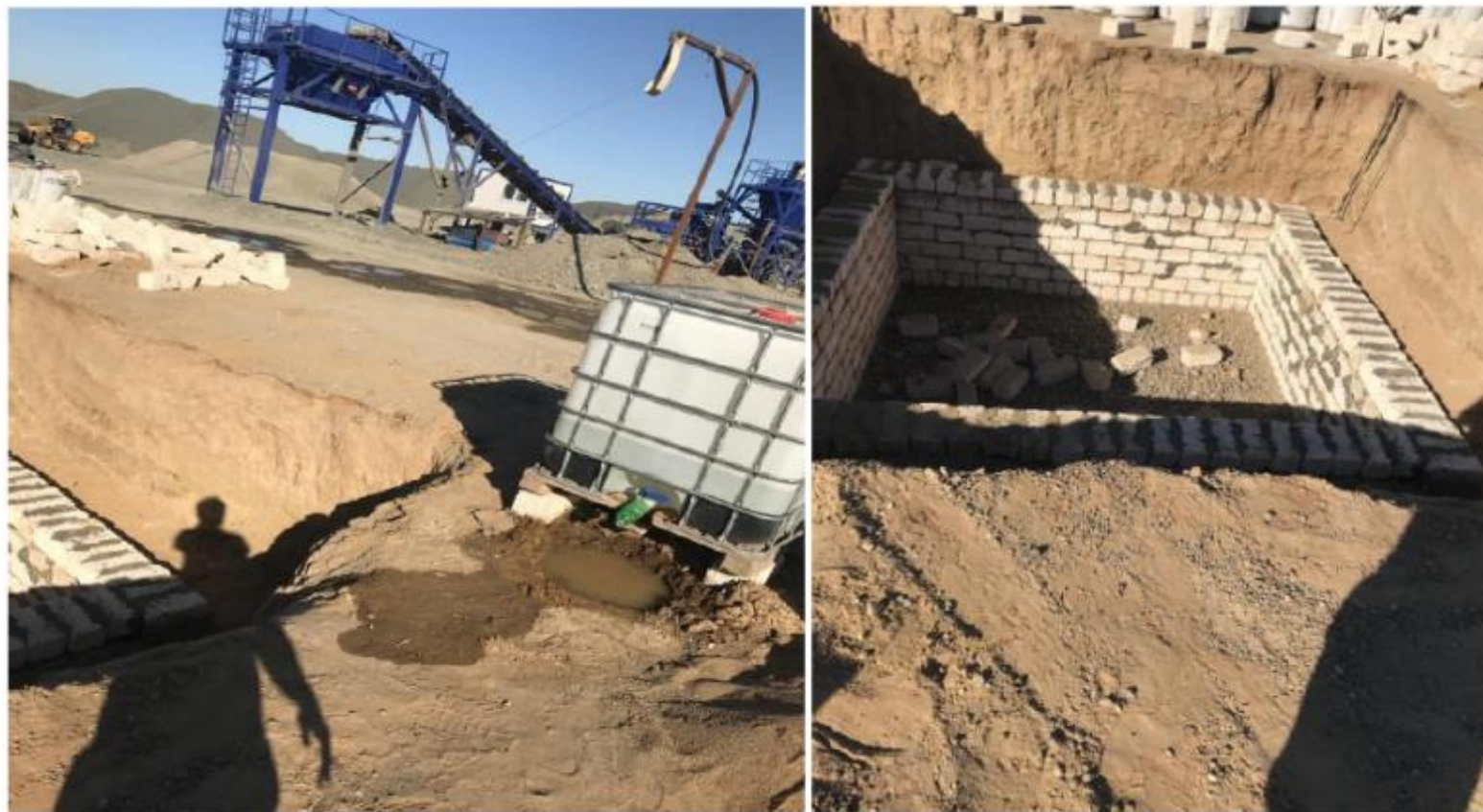
Lot 4 Construction of Storage Tank for Artesian Water, collecting at night time, for water trucks, dust control
